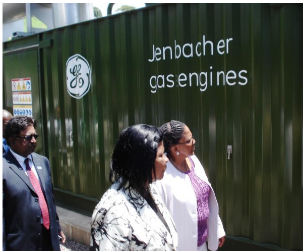
Minister's viewing containerised GE Jenbacher gas engines installed at Bisasar Road
